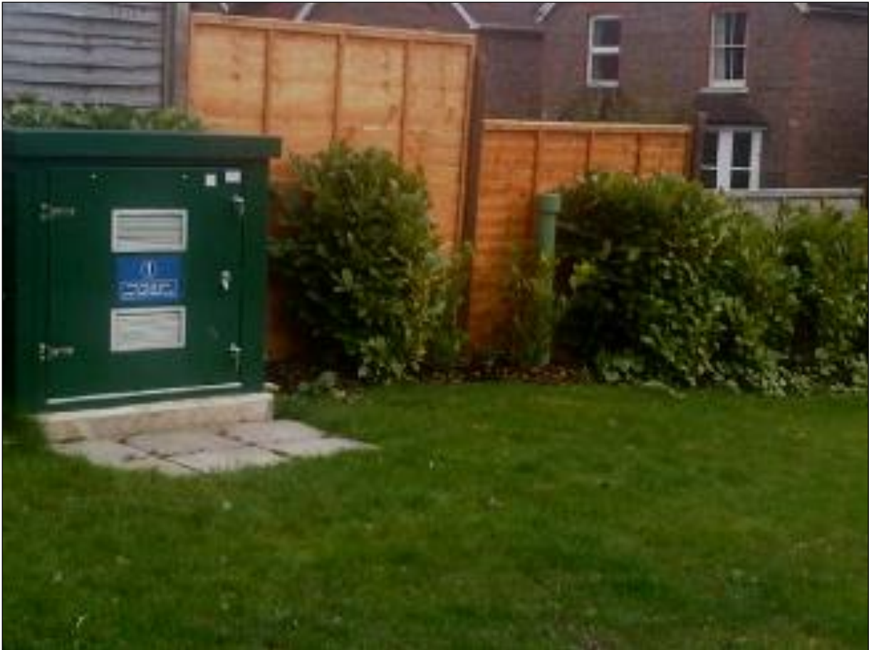
6 - Existing example of low level vent stack pumping stations
