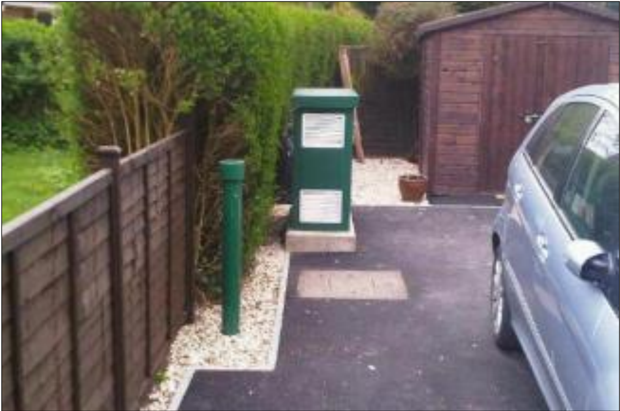
5 - Existing example of low level vent stack pumping stations
